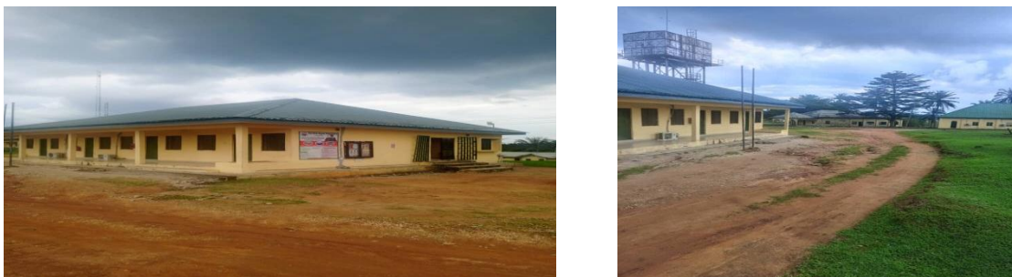
Fig. 10: The Head of Campus' Office Block calls for concern as the terrain is not users-friendly to people with mobility challenged. Source: Authors' Fieldwork, 2023
