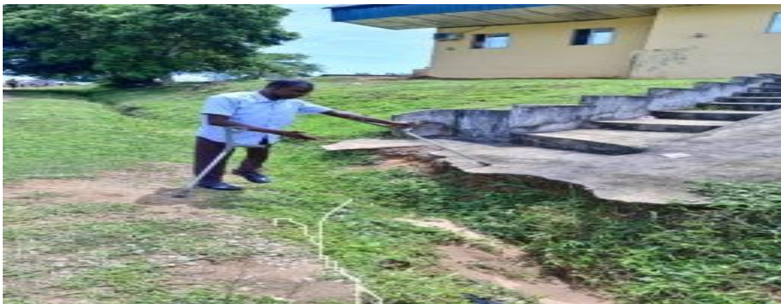
Fig. 14: Access to the Campus State-of- the- Art Pinnacle Theatre recommended for prompt intervention Source: Authors' Fieldwork, 2023
