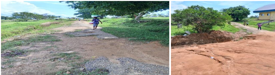
Fig. 13: Access to Centre for General Studies and Students' Affaires seriously threatened by erosion Source: Authors' Fieldwork, 2023
